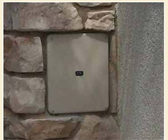
Required gas access panel
