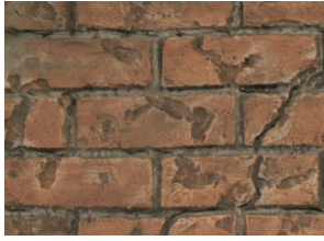
Fire Cracked Brick
